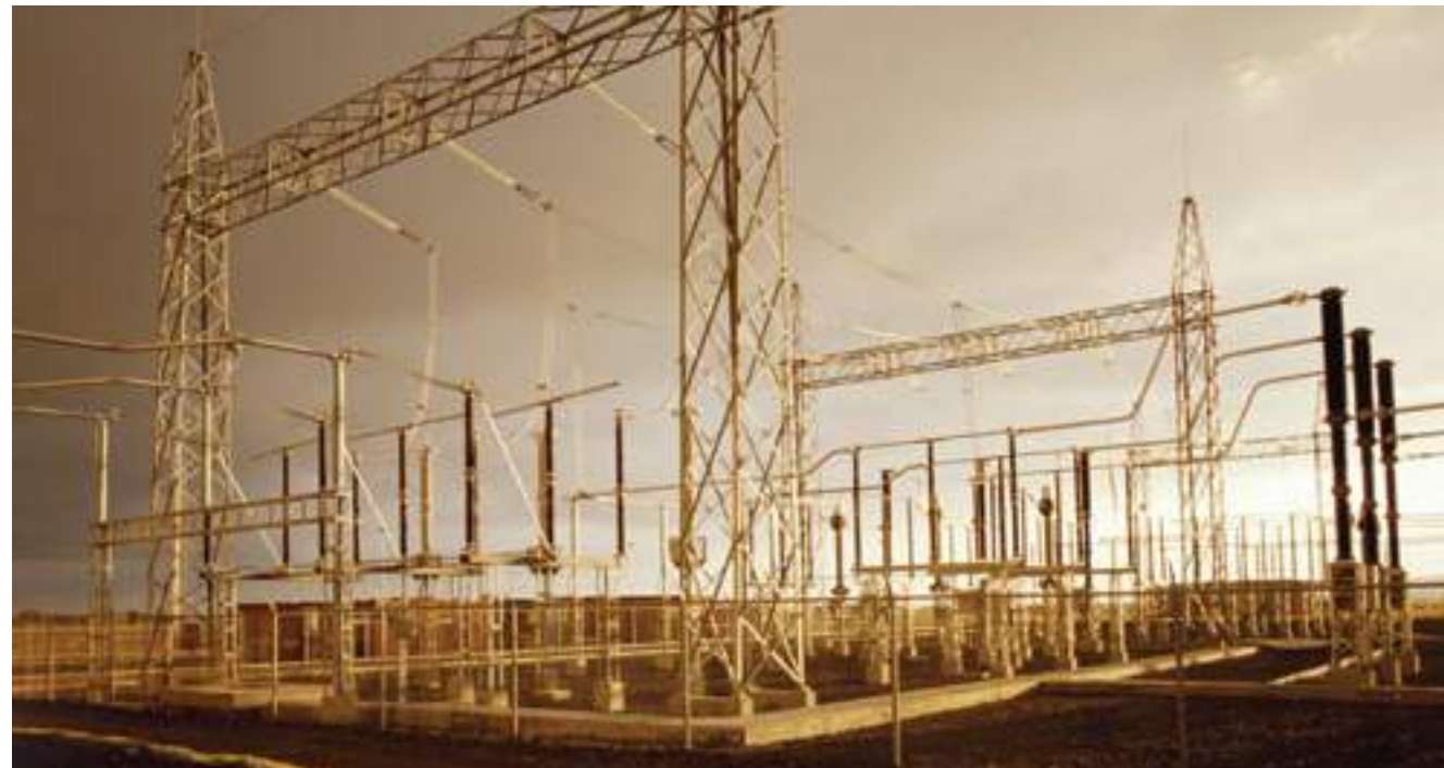
Pylons at a power generation plant.
