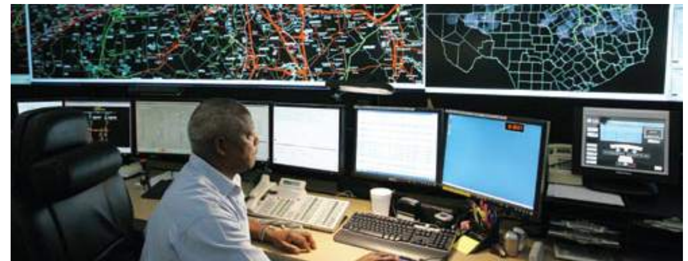
A transmission grid controller monitors grid performance from a control station.
